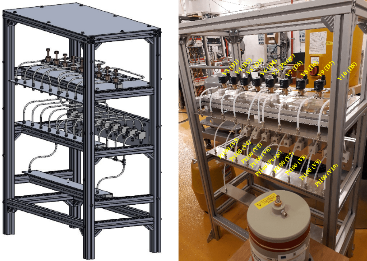
Figure 4.10.1: Design of the liquid nitrogen distribution panel (left panel) and the real assembly (right panel) of the system for cooling eight HPGe clover detectors, before the installation of the external thermal insulation wrapping.
